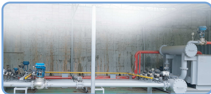
Flow and Flow Coefficient Test Equipment
